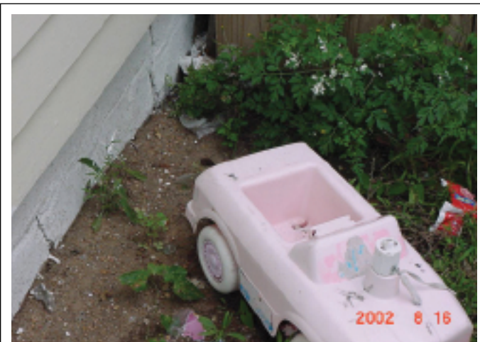
FIGURE 5.9 Soil lead hazard at dripline
