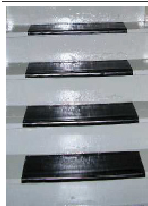
FIGURE 5.6b Friction hazard on stairs post-treatment.
