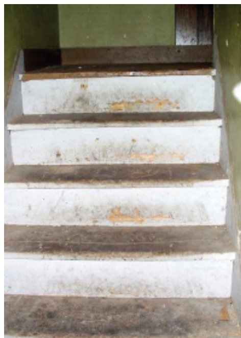
FIGURE 5.6a Friction hazard on stairs pre-treatment.
